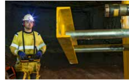
A handy remote radio control unit allows the driller to get a good view of the work area during critical positioning operations.
